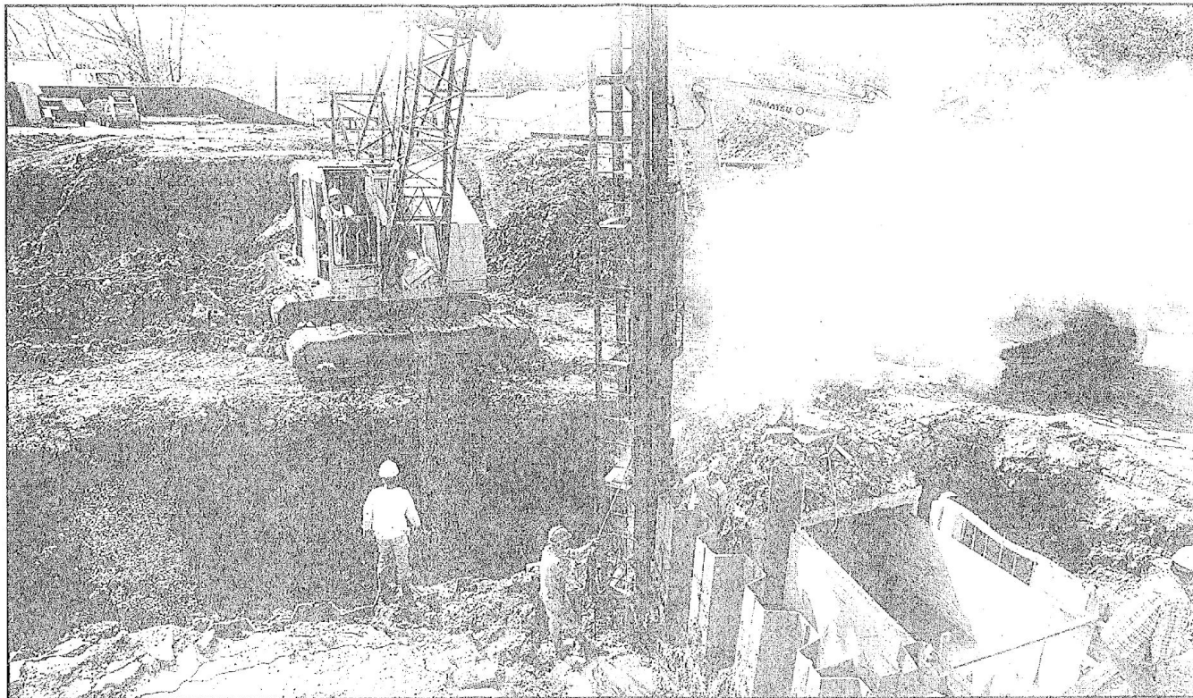
A Union Electric cleanup crew drives pilings to support a wall that will separate an area cleansed of carcinogenic coal tar from one that is not. (L.G. Patterson photo)
