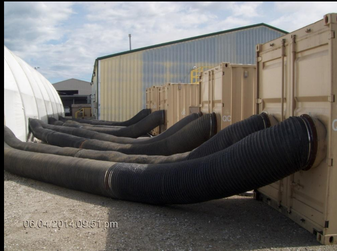
Granular Activated Carbon air treatment units
